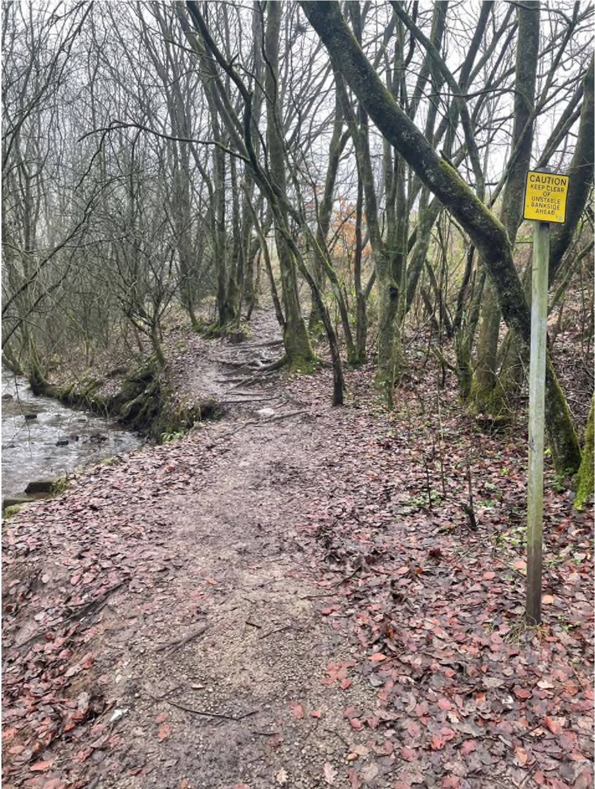
Photograph 15: Shows the route of footpath 26 going east from path routes from Ashbrook Road and sign which states "Caution Keep Clear of unstable bank side ahead"
